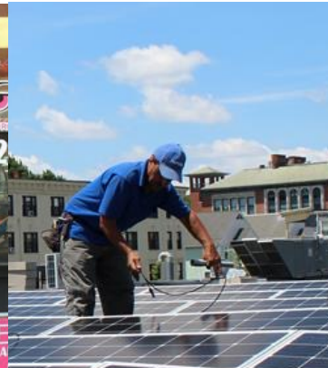
A worker installs solar panels at nonprofit-owned affordable housing - a strategy LISC supports through its STAR Solar initiative.
